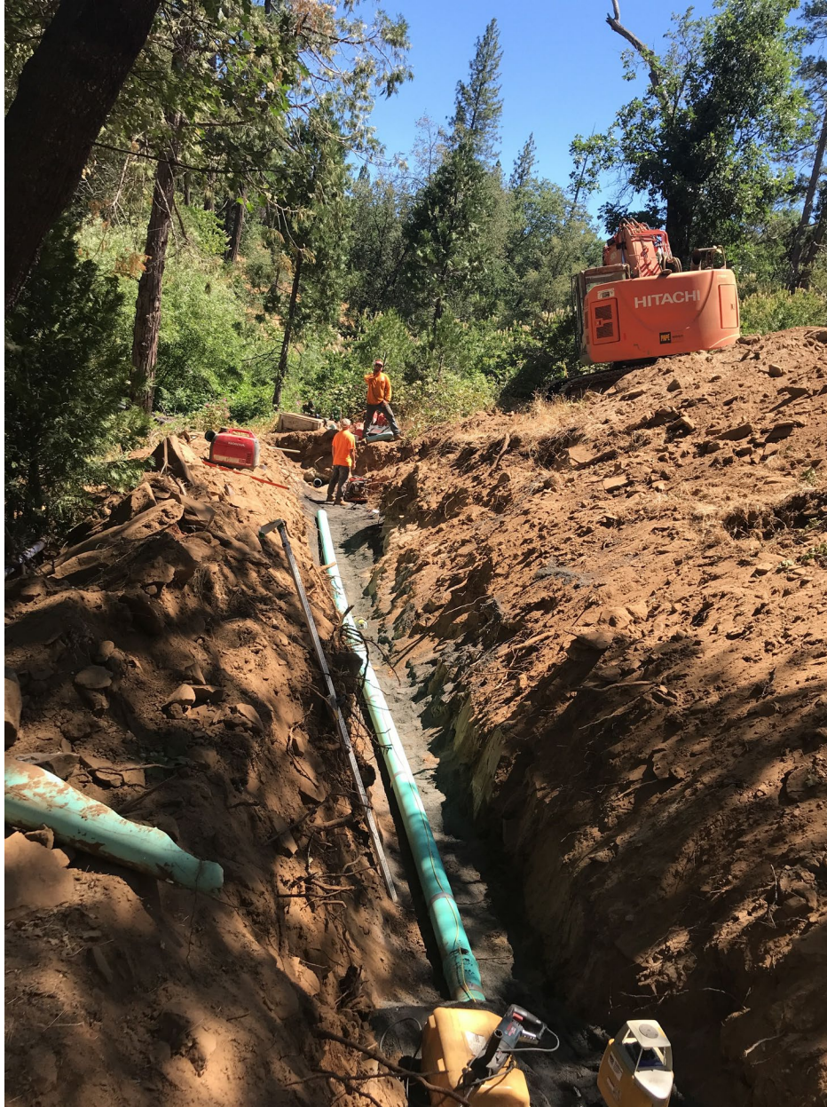
10 - Rehabilitate or Replace Approximately 11,500 feet of Failed Sewer Pipe
