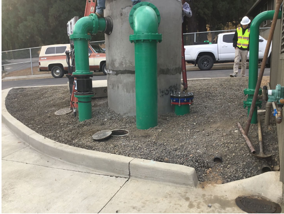
28 - New Influent Standpipe
