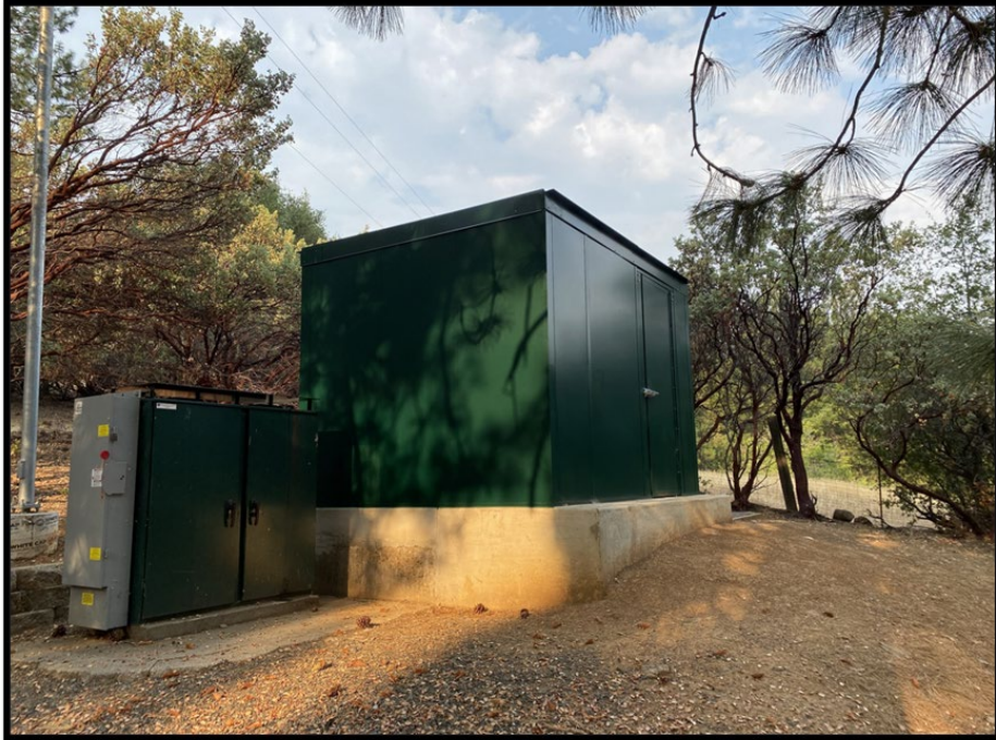
4 - Butler Wy After - Sound Enclosure
