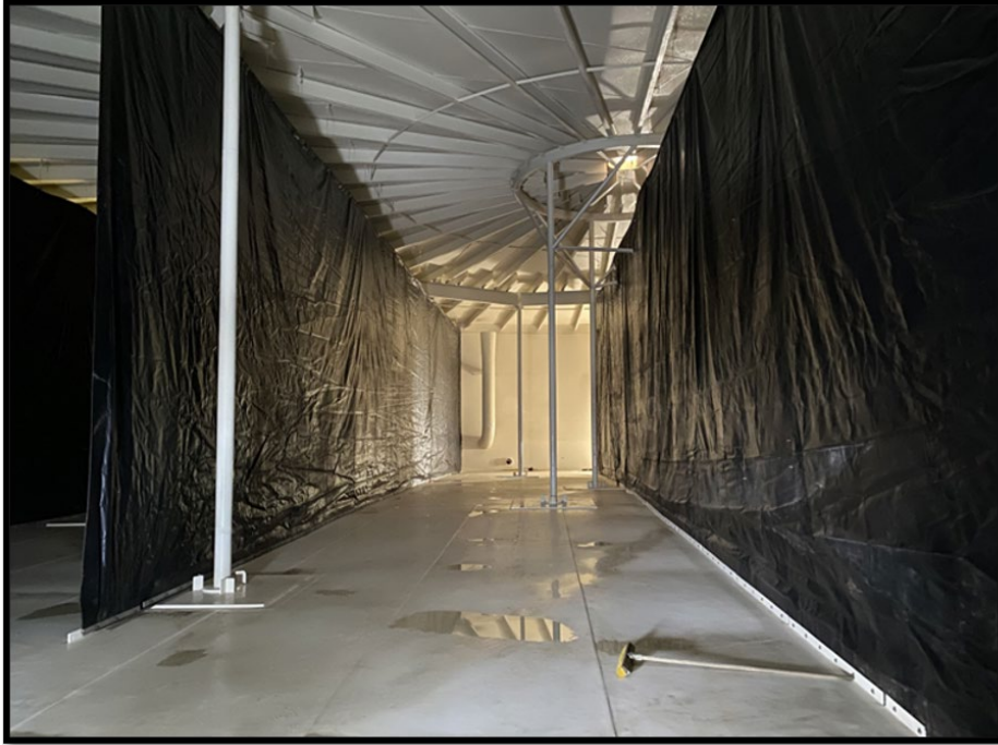
2 - After Sandblast, Structural Repairs and Recoating 2 Million Gallon Clearwells (Big Creek and 2G)
