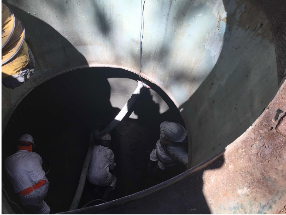
14 - Filled Bottom of Lift Stations With Concrete to Reduce Solid Accumulation and Reduce Odors
