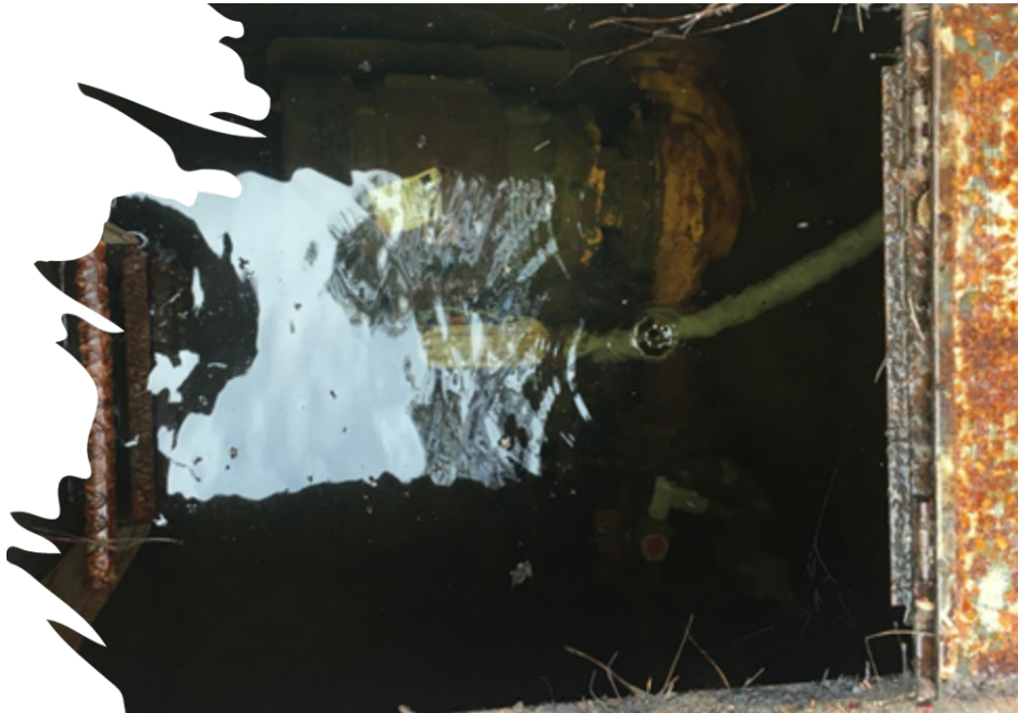
3 - Before - Butler Wy Booster Pump Underwater
